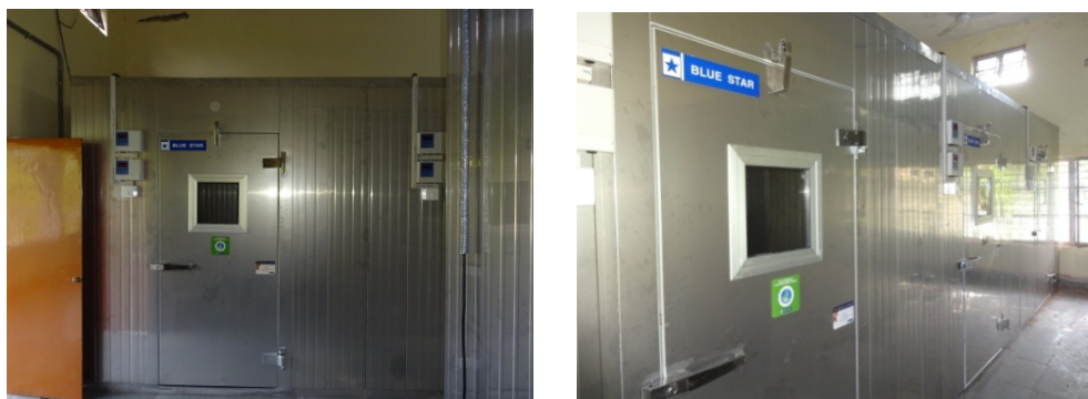
Newly installed Cold storage unit
