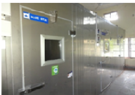
Cold storage facility at the institute
